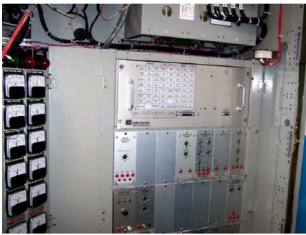
Figure 1: WDR-2000, showing voltage regulator and logic control modules
