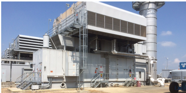
Figure 1. Typical MAVR-controlled combustion engine generator set
