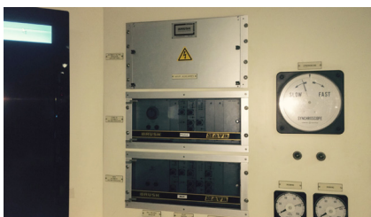
Figure 2. Redundant MAVR system with manual synchronization on the control panel
