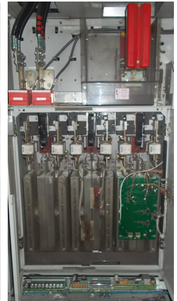
Figure 2: EX2000 Bridge Cubicle
