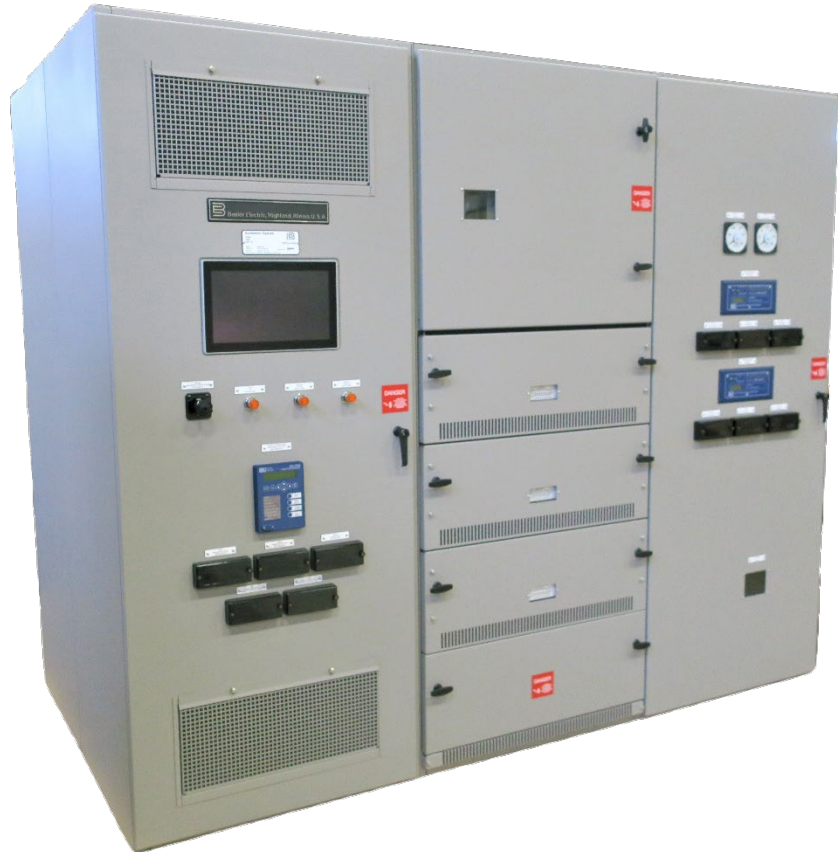
DECS-2100 System with N+1 redundancy
